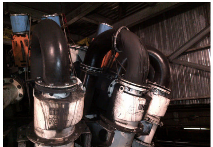
Cyclone Urethane Pipes
