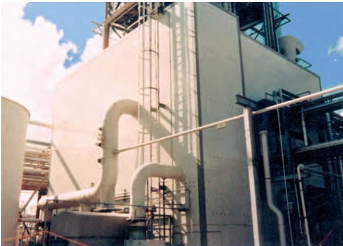
Airtight enclosure for Dow Chemical protects workers in adjacent areas against accidental escape of phosgene gas.
