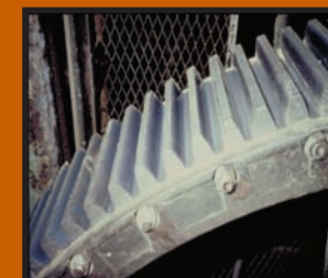
Pulp Mill Dryer Gears
